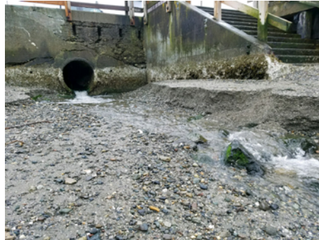
Existing Buried Redondo Creek Outfall
