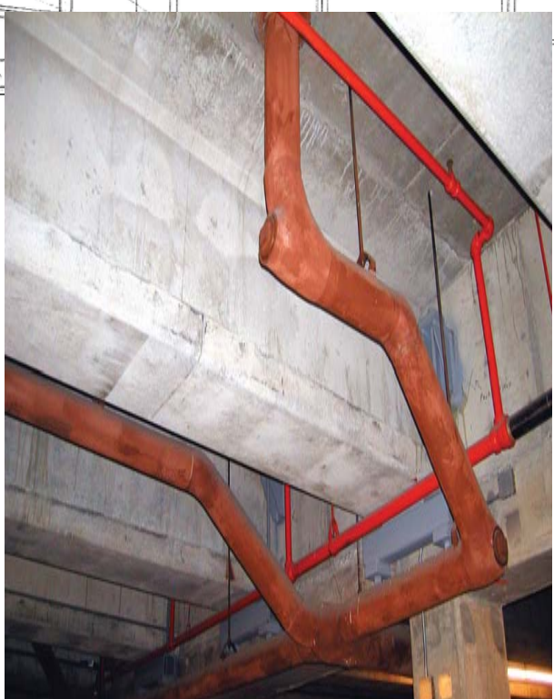
drainlines in garage
